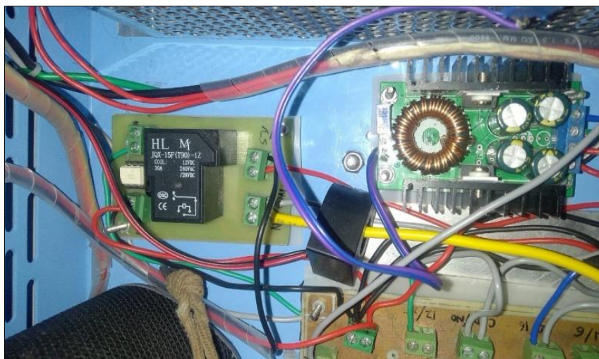
Fig. 10: Boost Converter and DC Relay
