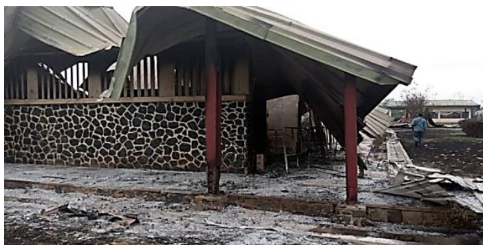
Picture 2: Remnants of the Mamfe District Hospital burned by unidentified armed men (08/06/2022) Source: Bisong Etahoben, Anglophone separatists in Cameroon raze Mamfe district hospital, retrieved from www.humanglemedia.com , on 27/08/2024 at 8:50pm
