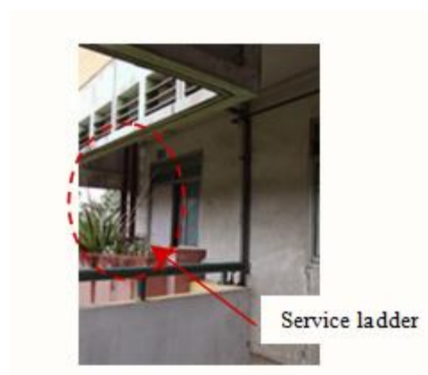
Fig-11: Position of service ladder
